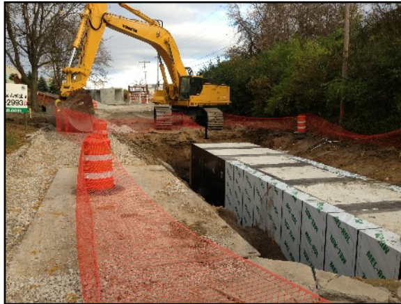
The “new” Bill Moose Run as it flows under a length of Freeway Drive.
